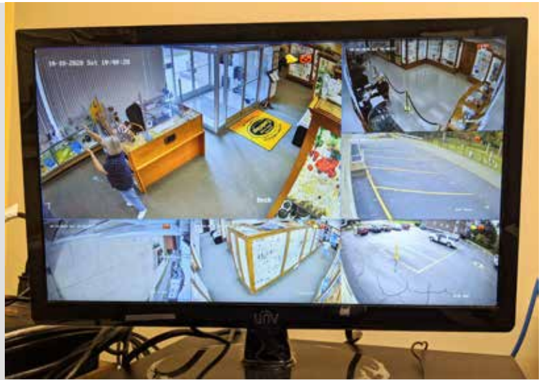
The museum’s security camera monitoring system “command central”. Up to 16 cameras can be added when funding becomes available.
